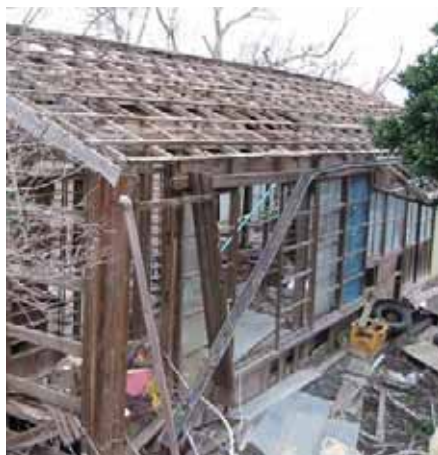
Roof Destroyed by Volcanic Gas
