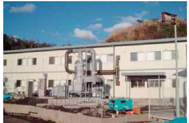
Desulphurization Equipment Installed in Accommodations
